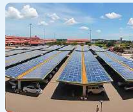
India's largest solar carport of 2.67 MW at Cochin International Airport Limited (CIAL)
