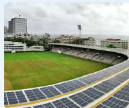
World's largest solar rooftop installation on a cricket stadium of 820.8 kWp at Cricket Club of India, Mumbai
