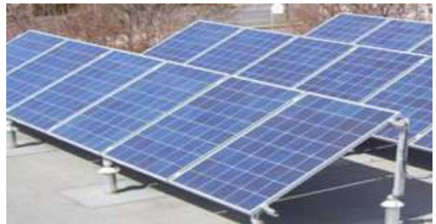
URJA SOLAR PV PANEL
