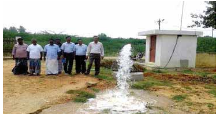
DRINKING WATER FACILITY AT DALAVOI
