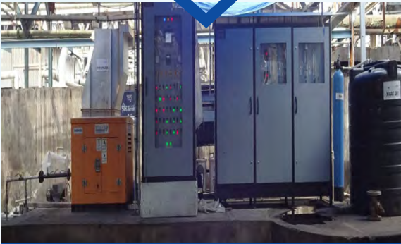
Electro-Oxidation Effluent Treatment Technology
