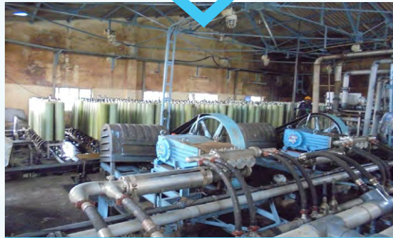
High Pressure Reverse Osmosis Plant at Nira
