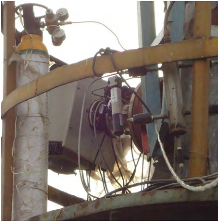
Online Stack Monitor at Gajraula
