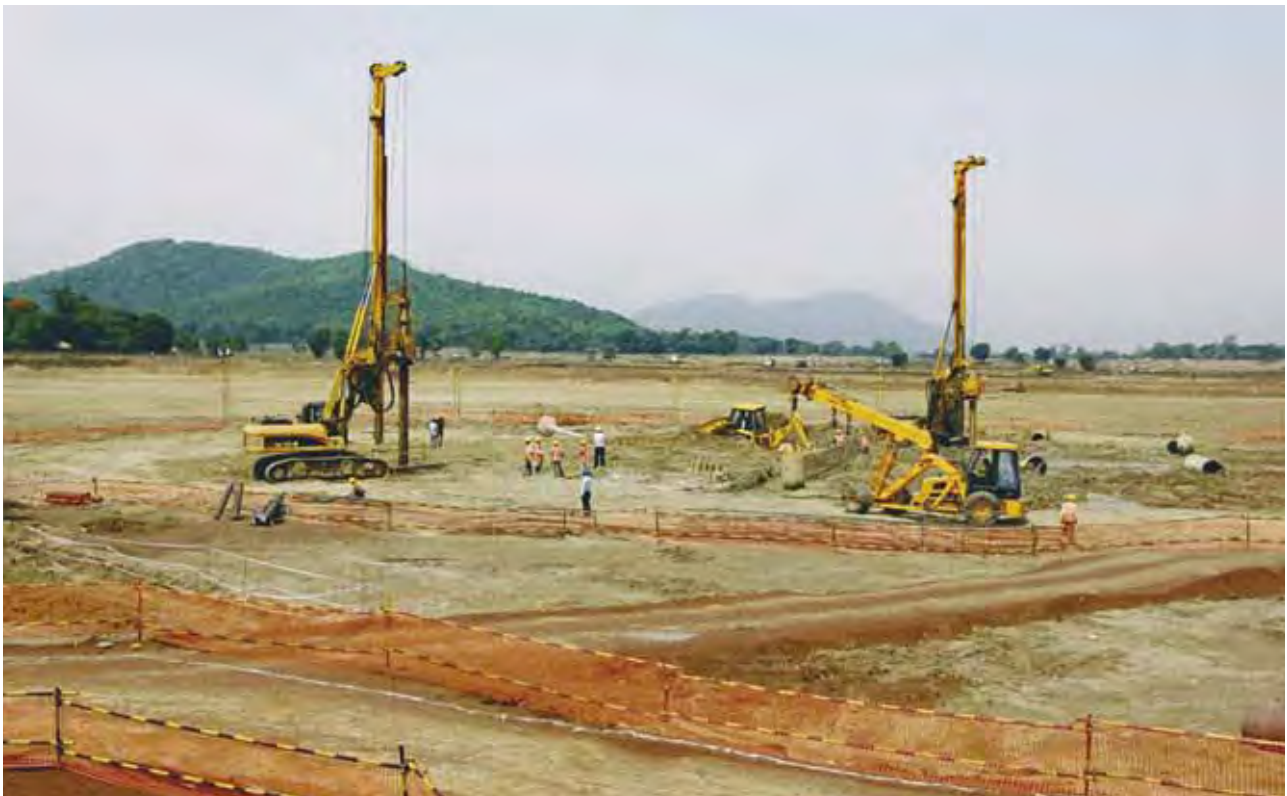
Piling work in progress at the proposed Blast Furnace site at Kalinganagar.
