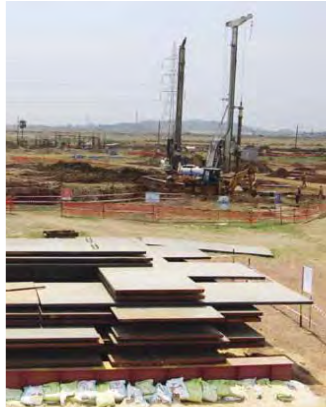
The Sinter Plant in its early stages of creation at the Kalinganagar site.
