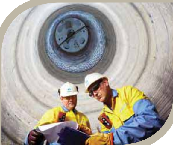
Inside the shell of the new No. 4 Blast Furnace at Port Talbot
