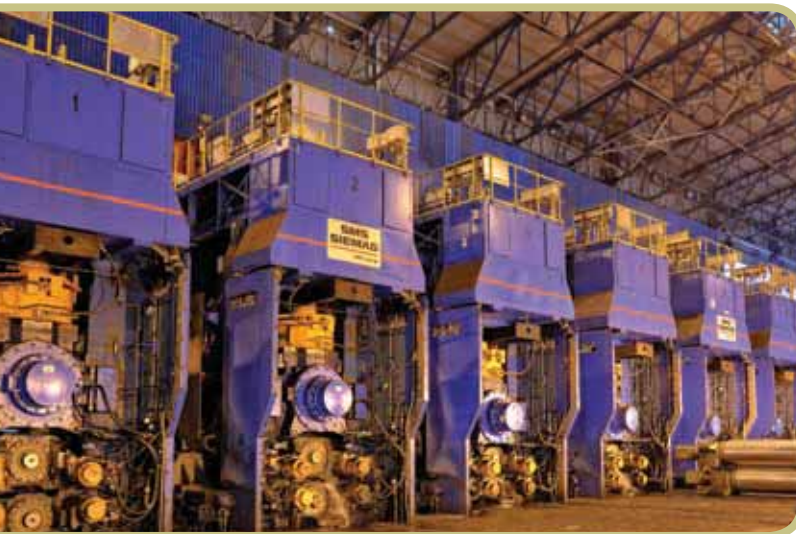
TSCR Facility at Jamshedpur Works
