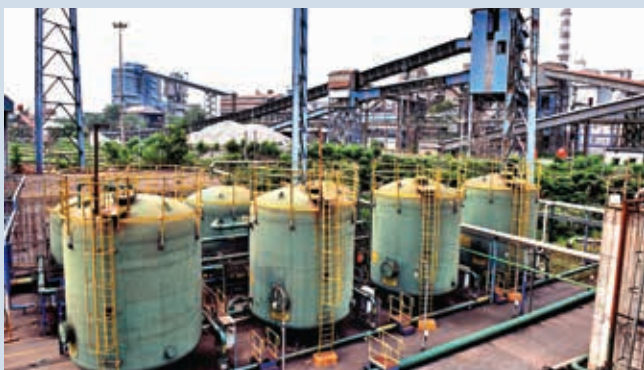
Central effluent treatment plant: Reducing water footprint
