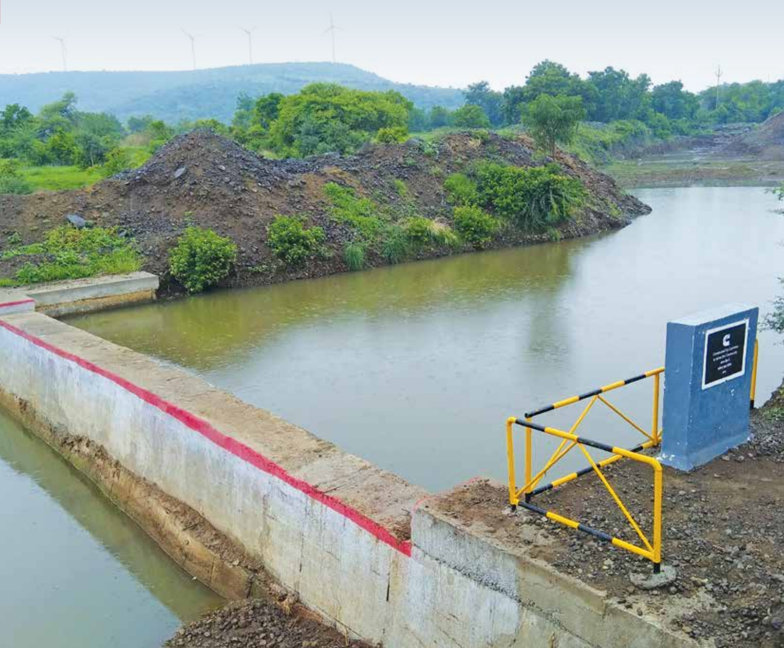
All for a greener world: Check dam constructed at Model Village Rajoda near Indore - one of the 12 Cummins model villages, conserving close to 14.3 million liters, supporting drinking water and agricultural needs of the village.
