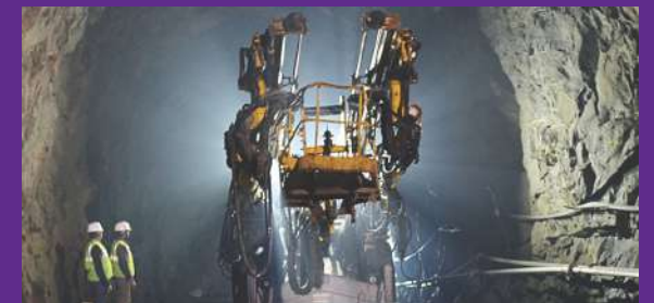
Kundah Hydroelectric Project, Tamil Nadu
