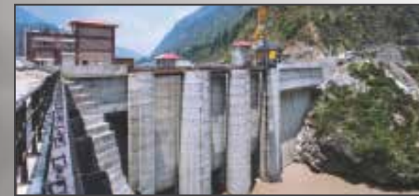
Parbati Hydroelectric Project, Himachal Pradesh
