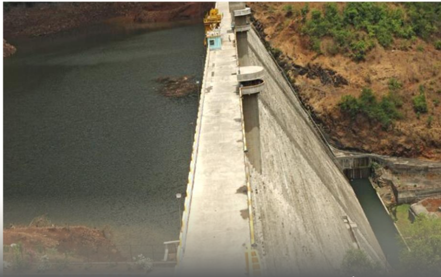
Ghatghar Dam – Maharashtra 84m high 10th fastest completed dam in the world an India's first RCC Dam
