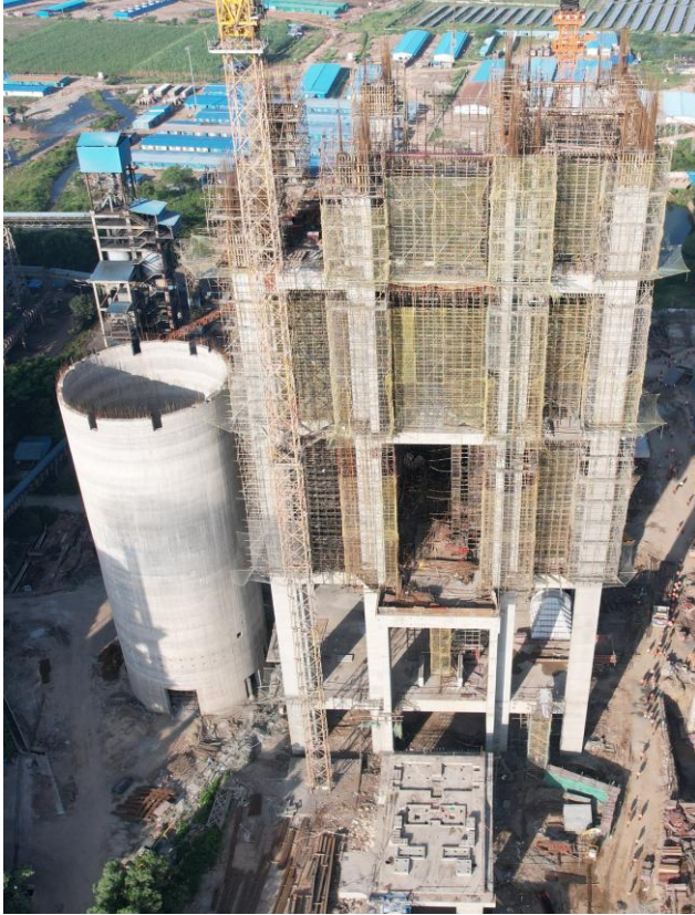
Preheater & Blending Silo
