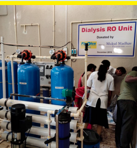
RO Unit at Civil Hospital Ratnagiri, Maharashtra
