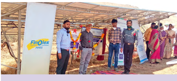
Solar water pump at Panawadi
