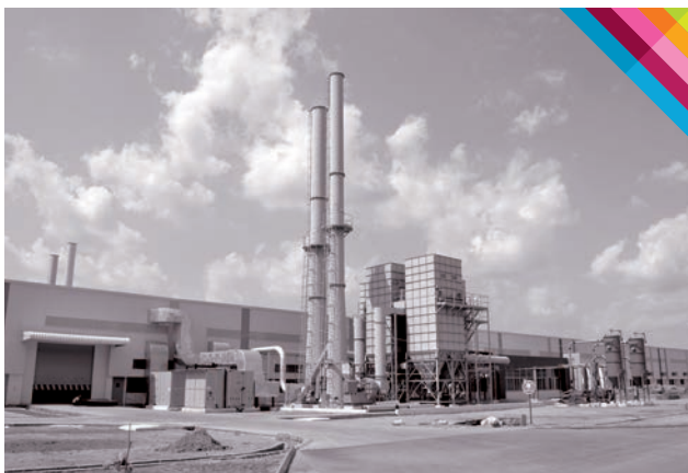
NEW DUST EXTRACTION, CENTRAL VACUUM AND FRESH AIR SYSTEMS FOR THREE ASSEMBLY LINES AT THE NUNEGUNDLAPALLE VILLAGE, CHITTOOR DISTRICT.
