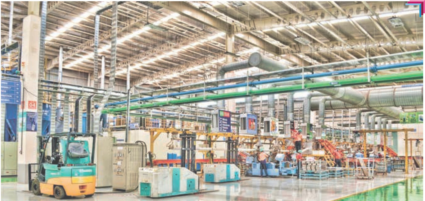
Automotive Battery facility at Nunegundlapalle Village, Chittoor District
