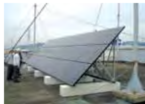
4kW Standalone Solar installation, Japan
