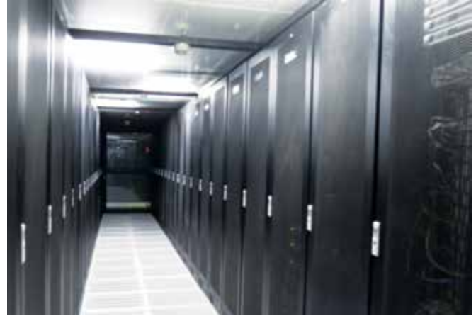
RailTel Data Center at Gurugram
