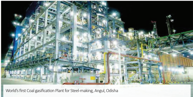
135X6 (810) MW Captive Power Plant, Angul, Odisha
