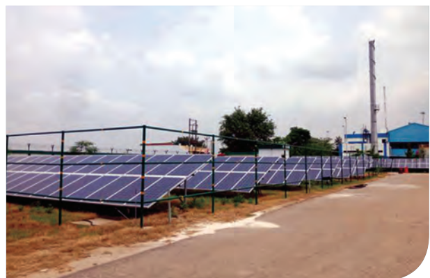
130 KWp Solar Power plant at Industrial Packaging, Asaoti
