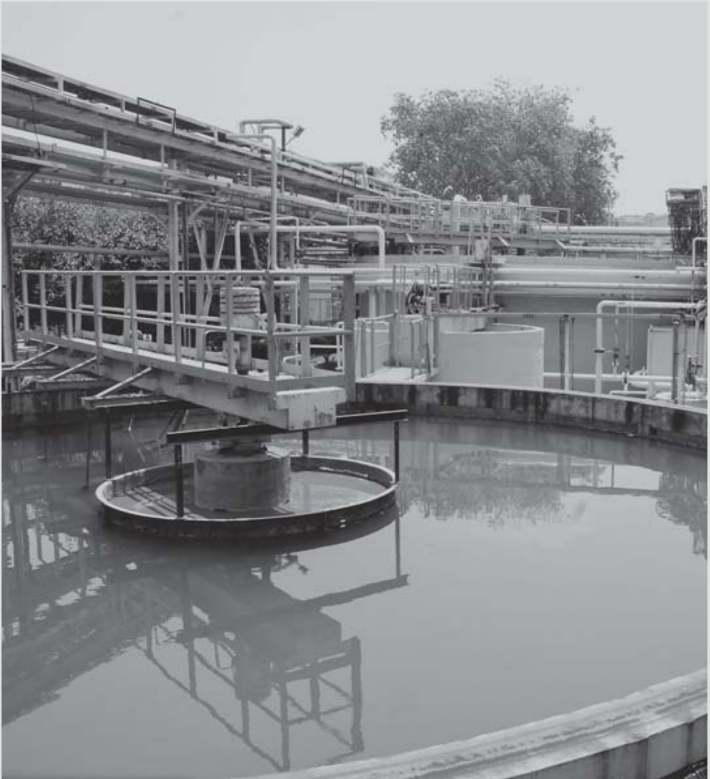
Effluent Treatment Plant at the Gurgaon facility.
