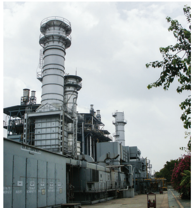
Natural gas based captive power plant at Gurgaon facility
