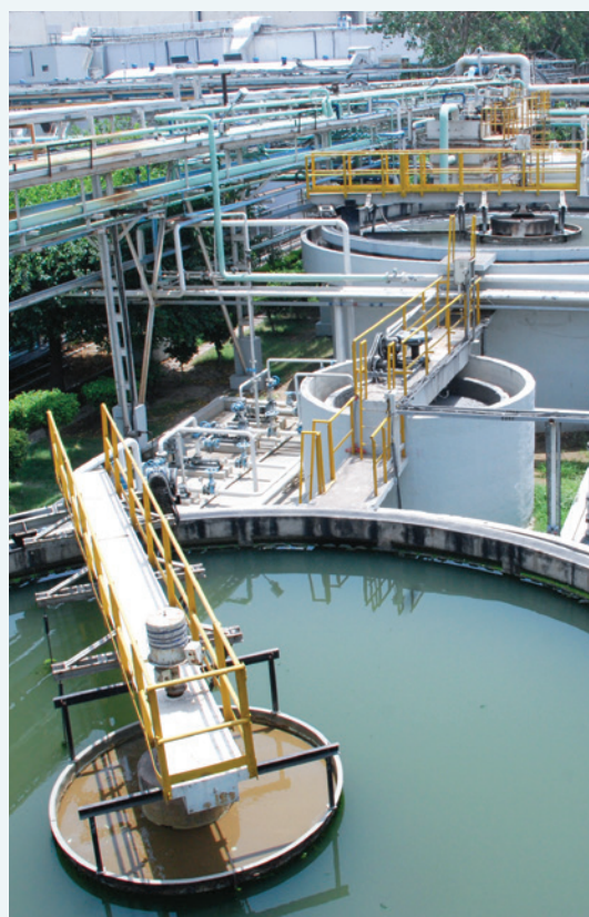
Effluent treatment plant at Gurgaon facility
