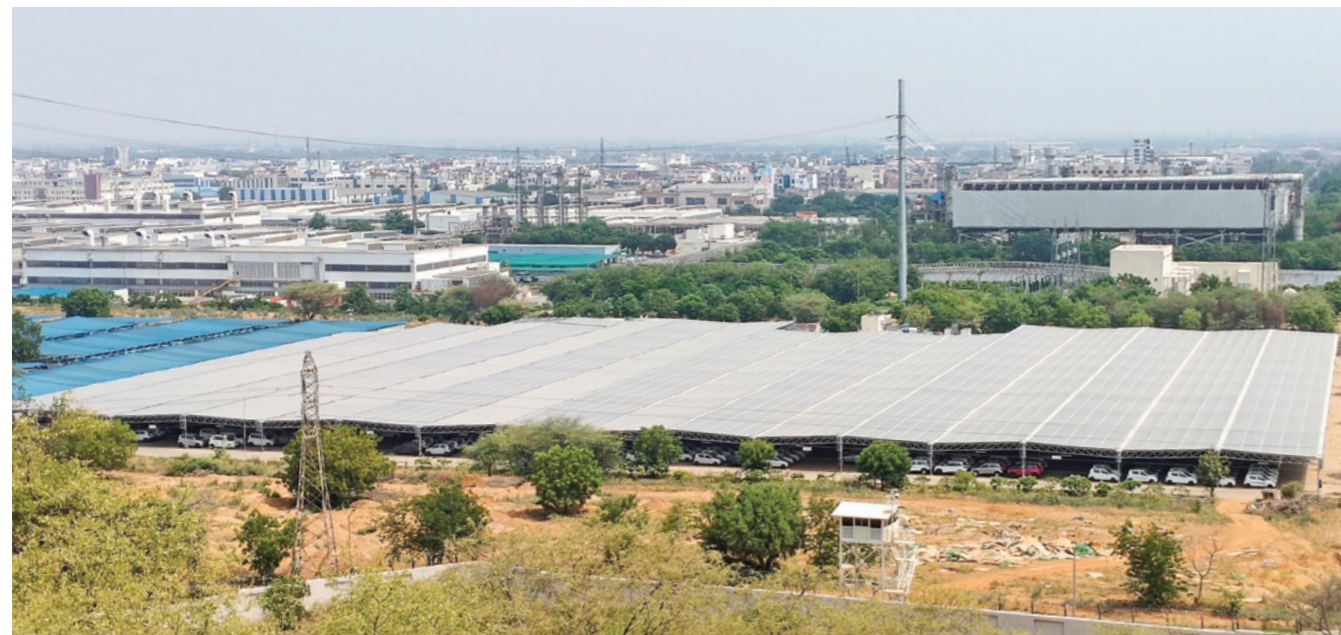
New solar plant at Manesar facility
