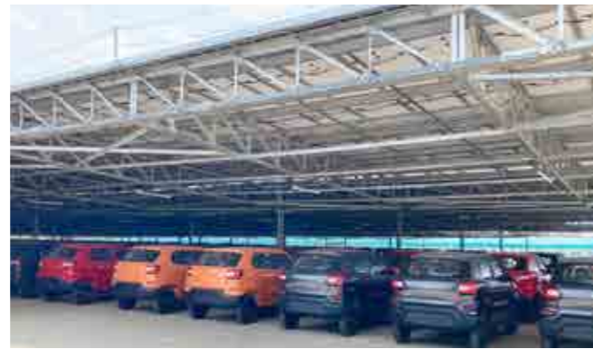
Carport Type Solar Power Plant (bottom view)
