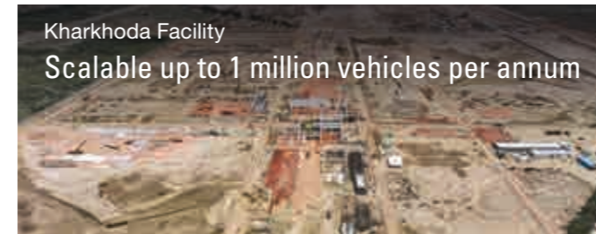
Kharkhoda manufacturing facility construction in progress. First plant to be commissioned in 2025.
