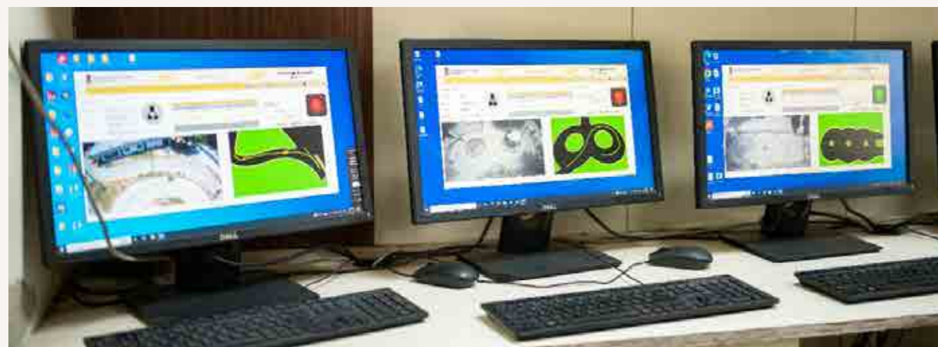
Computer center with automation software
