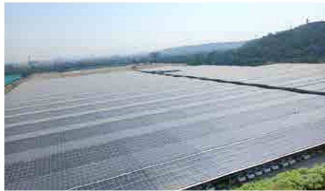
Carport Type Solar Power Plant (top view)
