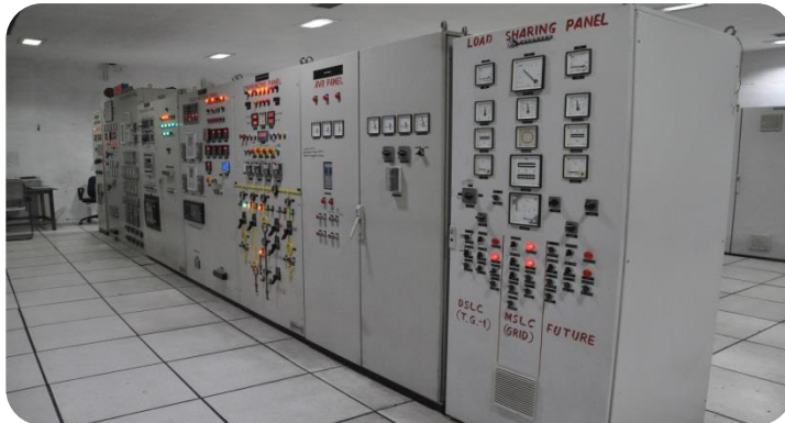
Cogeneration Control Panel
