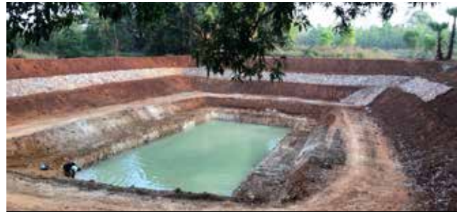
Water harvesting structures for livelihood improvement by double cropping & cash crops, Ghodabara, Odisha
