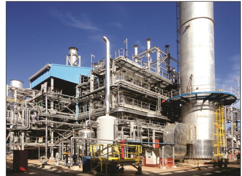
Oil & Gas Fired Boiler
