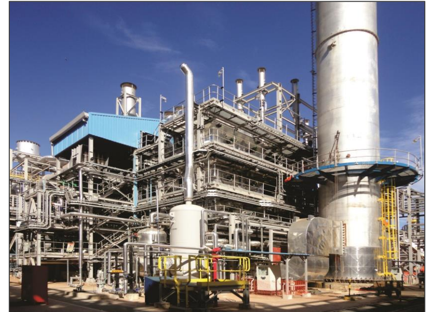
Oil & Gas Fired Boiler
