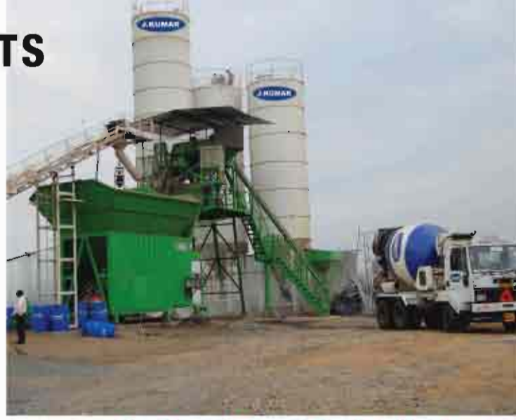
Readymade Concrete Mix Plant
