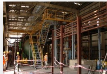
COLOUR COATING LINE FOR TATA BLUESCOPE LTD.
