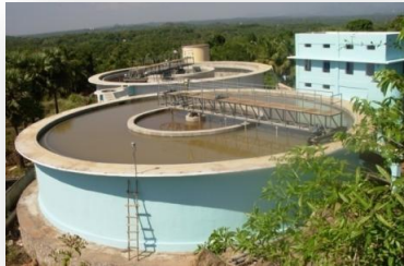
WATER TREATMENT FOR TWAD BOARD
