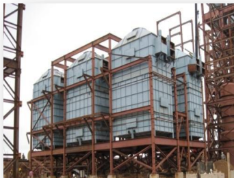
COAL GASIFICATION PLANT FOR JINDAL STEEL
