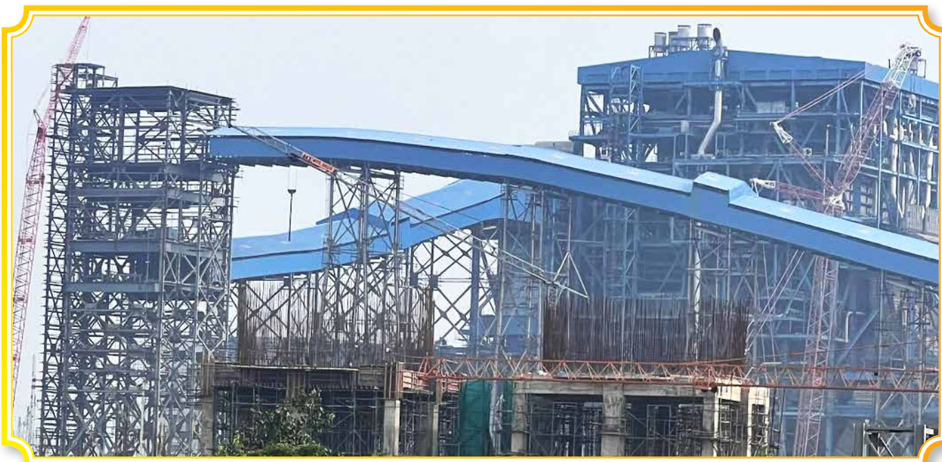
2x660 MW Buxar Thermal Plant, Bihar financed by REC
