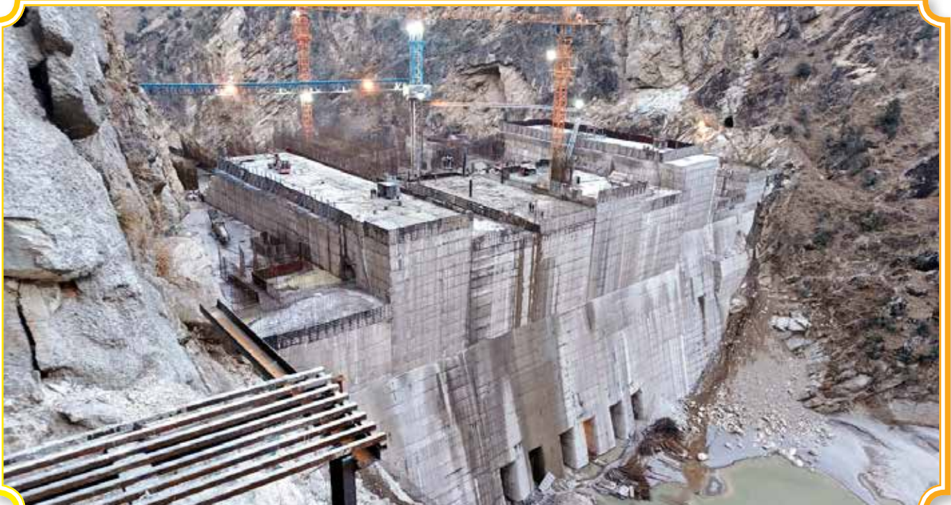
624 MW Kiru Hydro Electric Plant, Jammu & Kashmir financed by REC
