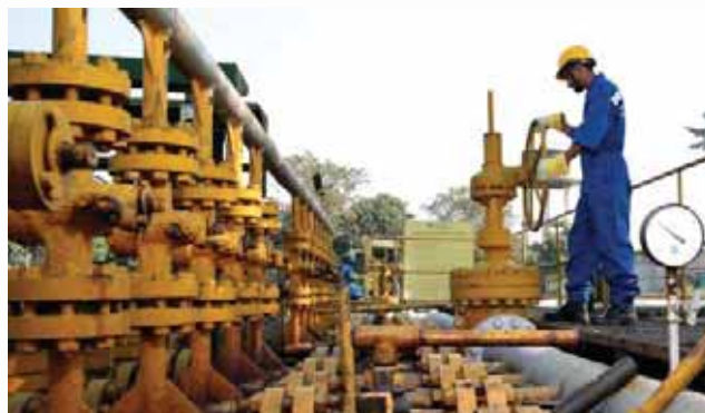
View of a Natural Gas Installation at Fields Headquarters
