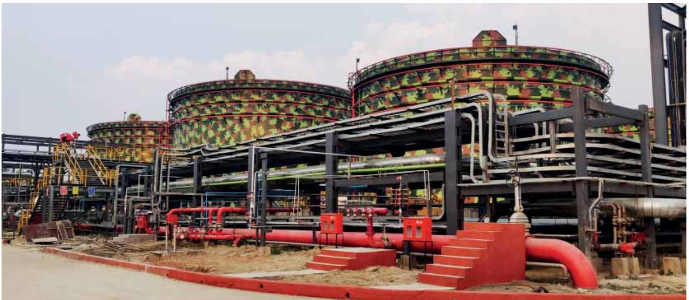
View of Secondary Tank Farm in Dibrugarh inaugurated by Hon'ble Prime Minister in February 2021
