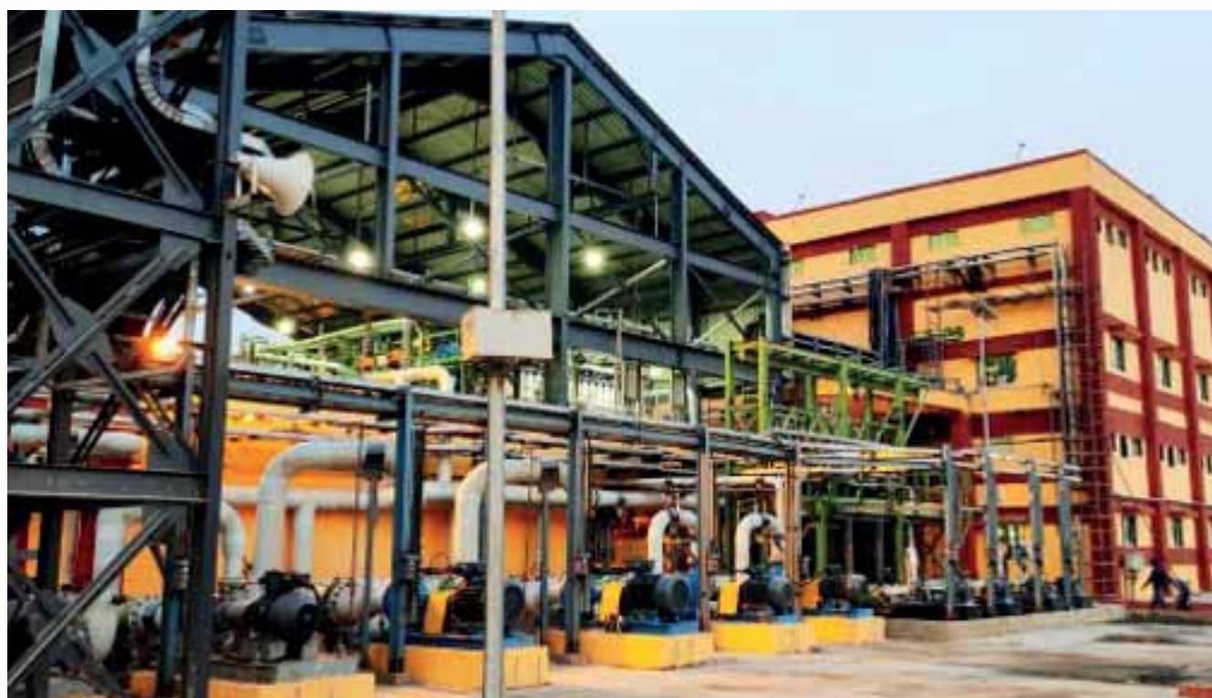
View of Secondary Tank Farm in Madhuban, Dibrugarh inaugurated by Hon'ble Prime Minister in February 2021
