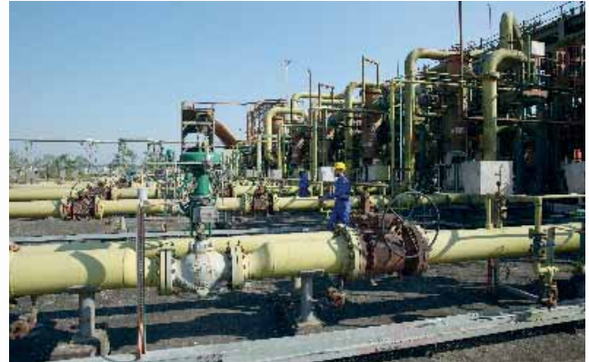
View of Natural Gas Installation at OIL's Field Headquarters, Duliajan
