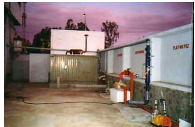
Harvesting facilities at units
