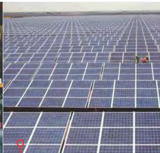
Module Mounting Structures- Gujarat Solar Park
