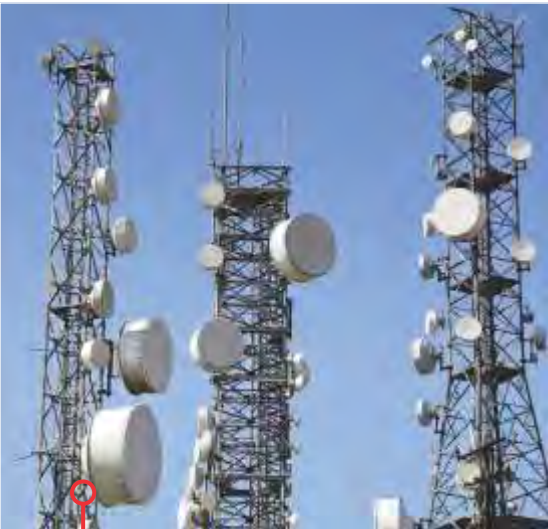
Telecom Tower Structure
