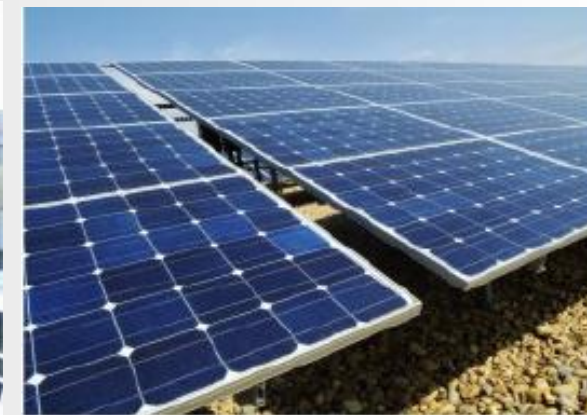
Module Mounting Structures- Gujarat Solar Park
