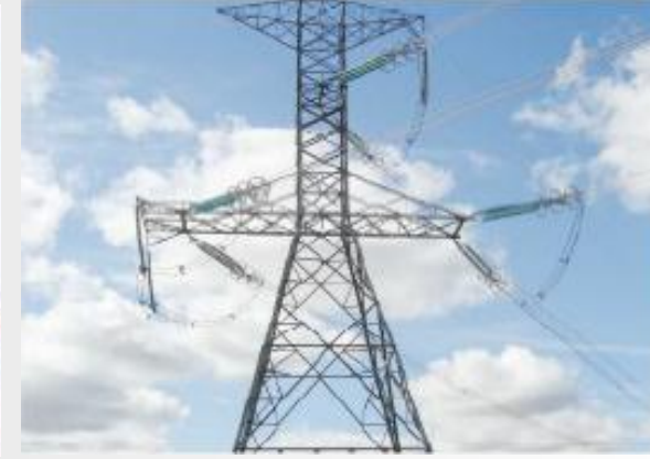
Substation Tubular Structure- Powergrid Corporation Ltd.
