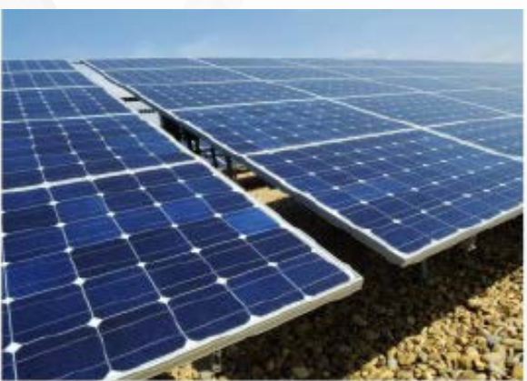
Module Mounting Structures- Gujarat Solar Park
