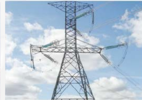
Substation Tubular Structure- Powergrid Corporation Ltd.
