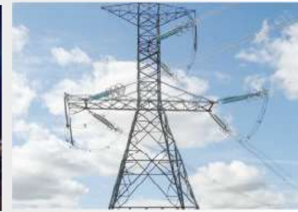
Substation Tubular Structure- Powergrid Corporation Ltd.
