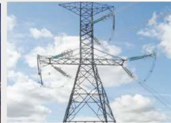
Substation Tubular Structure- Powergrid Corporation Ltd.
