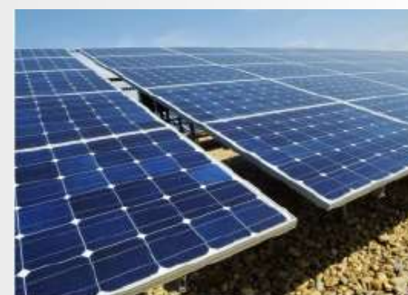
Module Mounting Structures- Gujarat Solar Park
