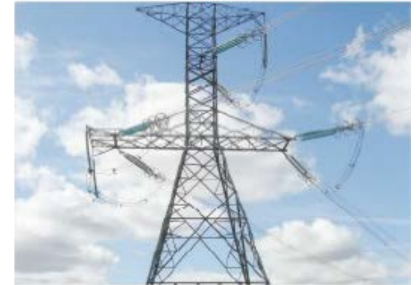
Substation Tubular Structure- Powergrid Corporation Ltd.
