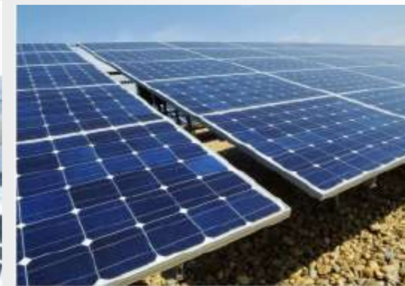
Module Mounting Structures- Gujarat Solar Park
