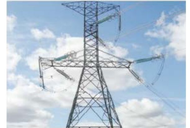
Substation Tubular Structure- Powergrid Corporation Ltd.
