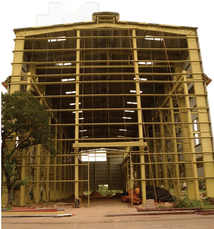
Civil and allied works in Progress for erection and installation of 20 T capacity Electric Arc Furnace
