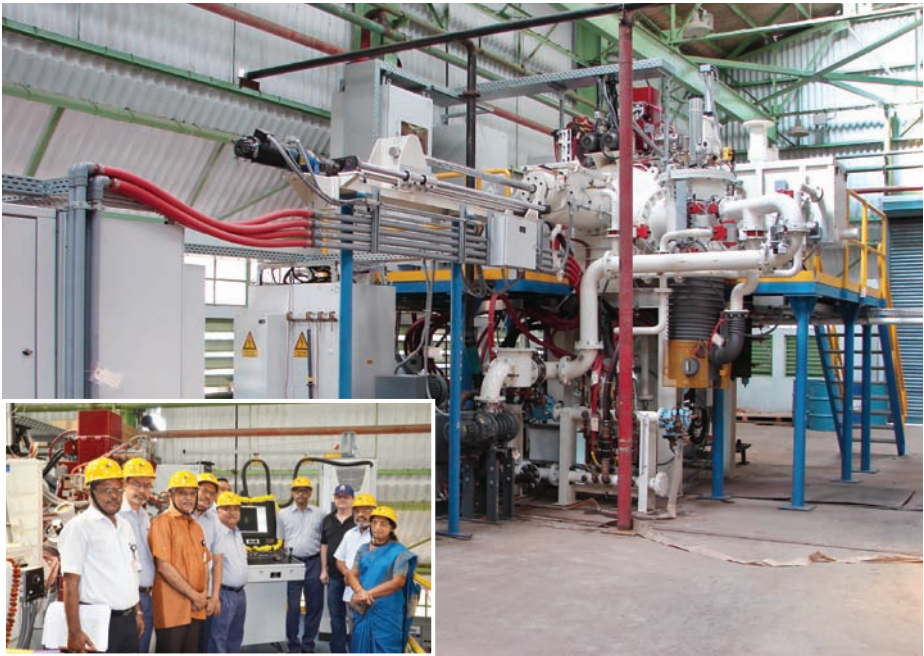
The newly commissioned Electron Beam Melting furnace. (Inset) MIDHANI functional Directors with representatives from VSSC during Inauguration of the Furnace
