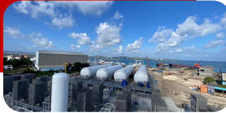
Order received for LNG regassification for two small Islands, Abaco & Eleuthera of The Bahamas, for power generation facilities
