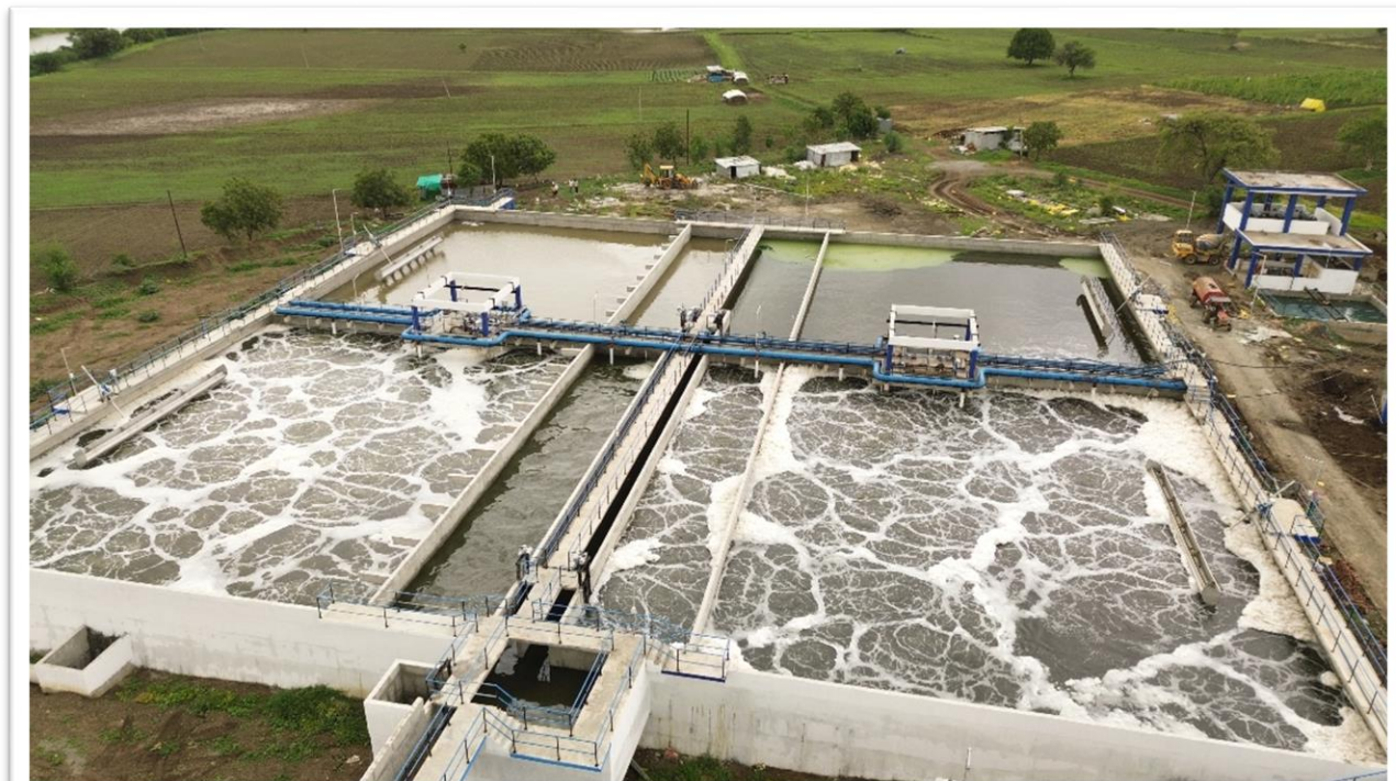
32 MLD STP Plant at Latur, Maharashtra
