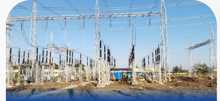
220 kV Power arrangement for Grasim from GETCO
