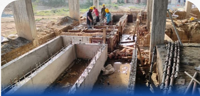
132 kV GIS at Lalsagar, Jodhpur
