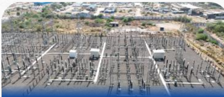
66 kV Power arrangement at GIDC Saykha (Private)
