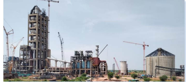
Nagaur IU – pyro processing and clinker silo
