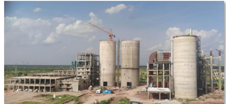
Nagaur IU – cement grinding and packing & dispatch
